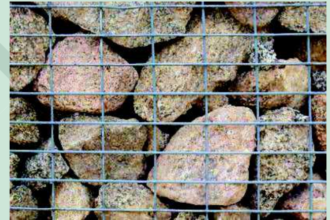
Figure 13. | gabion cages with local stone used for waterside retaining (pennant or limestone)
